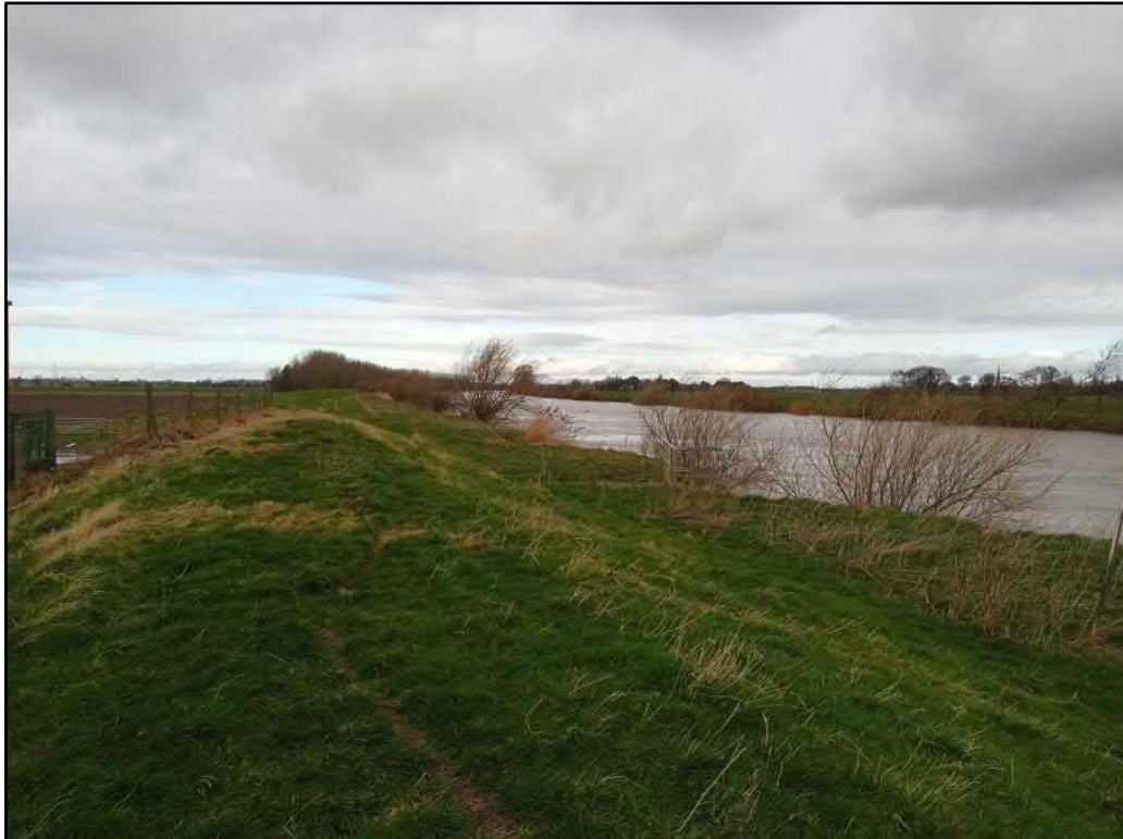
Plate 0.8 - Picture of the flood defences of the River Ouse taken during site visit undertaken on 22 February 2022
